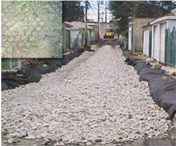
The alley, constructed of a rigid grid system and gravel, allows rainwater to soak into the ground. Close up of finished system upper left corner.
